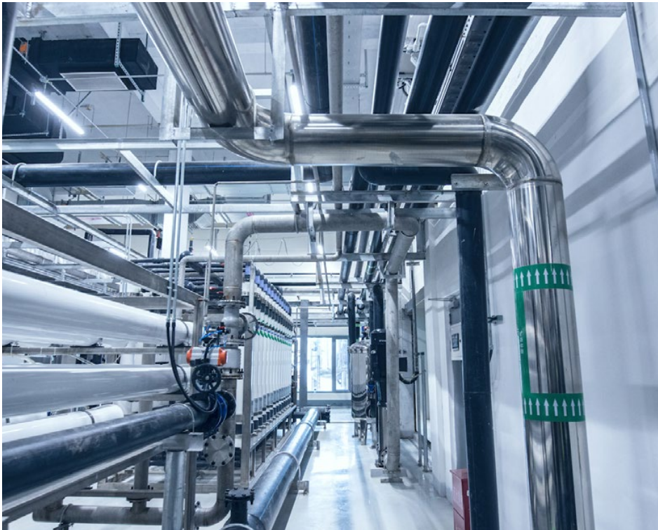
Interior view of the reclaimed water station
