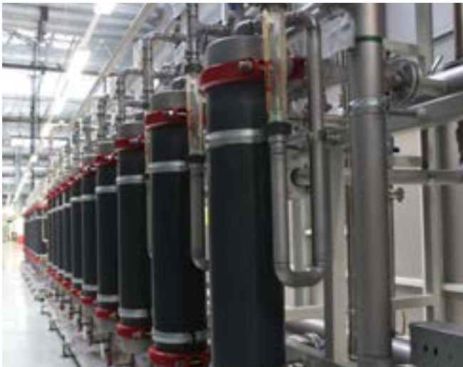
Our electrocoating ultrafilter system reduces wastewater discharge.
